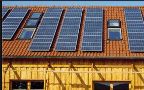
Photovoltaic panels on house roof
